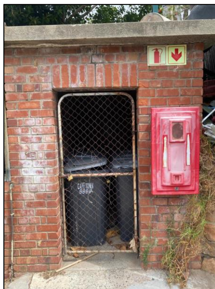
Figure 5. Well-secured waste at Miller's Point Resort.
